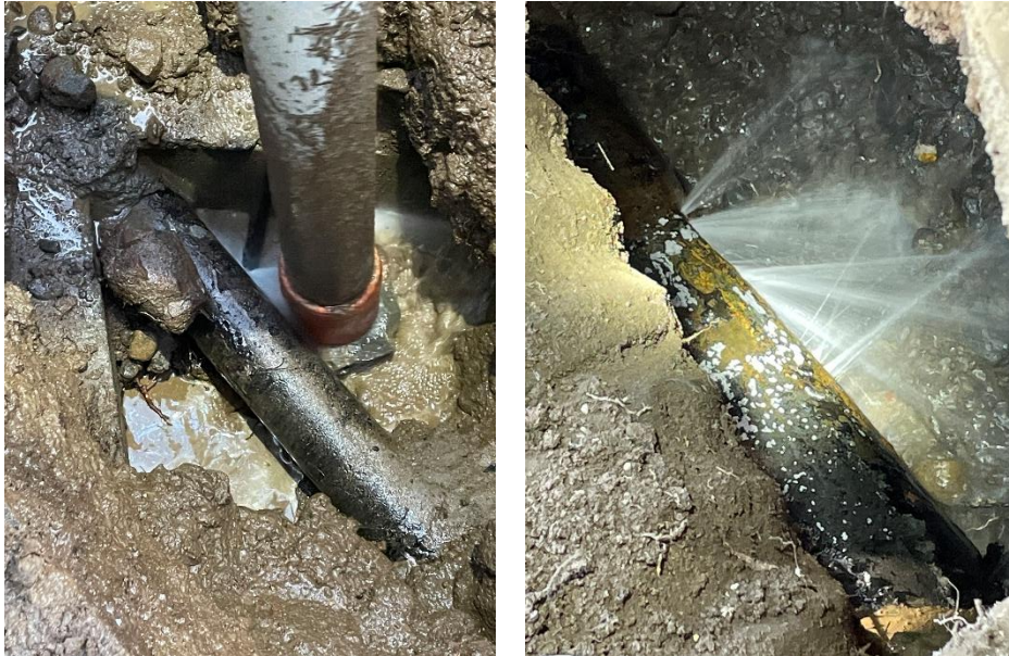
Figure 2 Pictures of different leaks experienced over the past few weeks. The crews have been responding to leaks quickly to minimize water losses.
